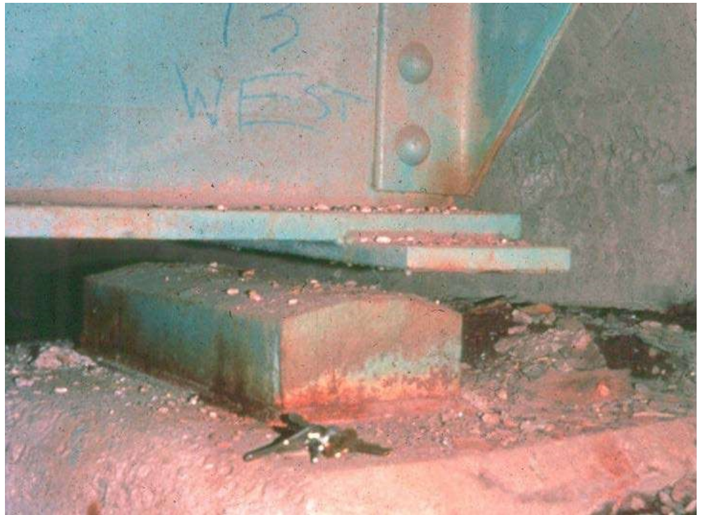
Figure 11.1.31 Uplift at Bridge Bearing
