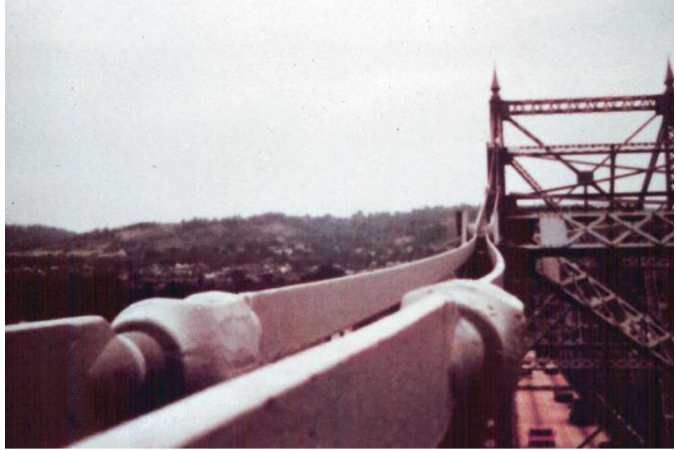
Figure 10.9.21 Bowed Eyebar Member
