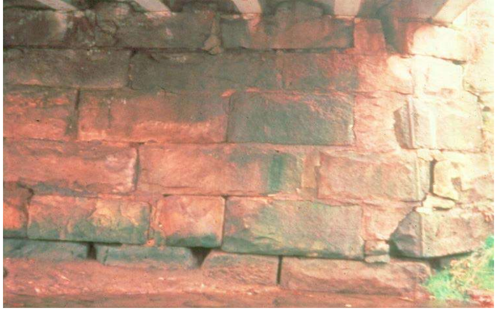
Figure 12.1.34 Stone Masonry Abutment with Deteriorated Joints
