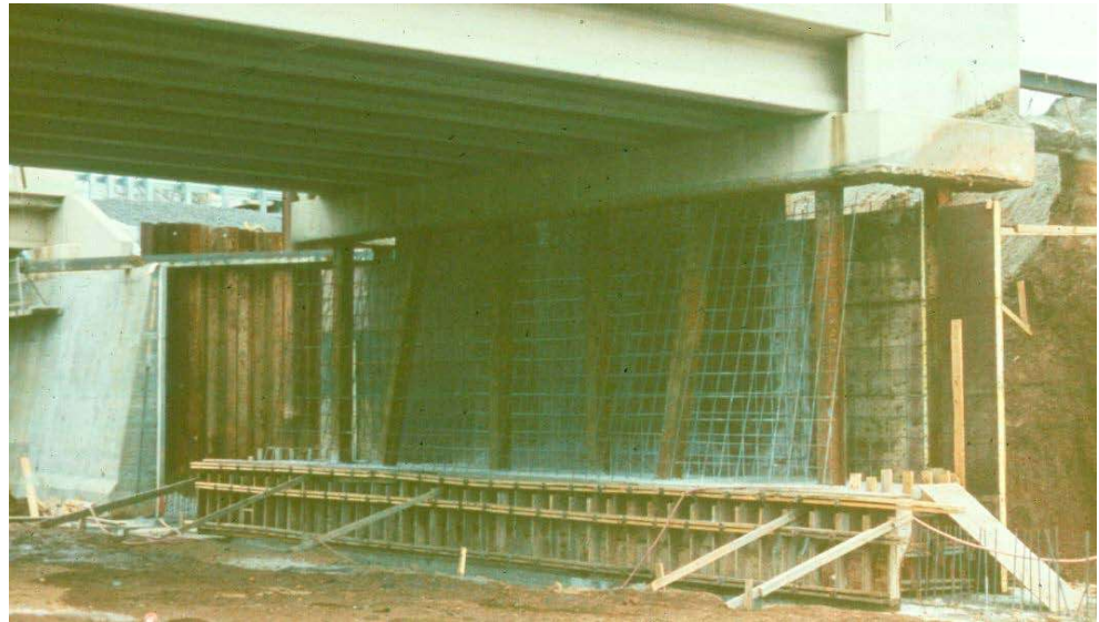
Figure 12.1.22 Stub Abutment on Piles with Piles Exposed
