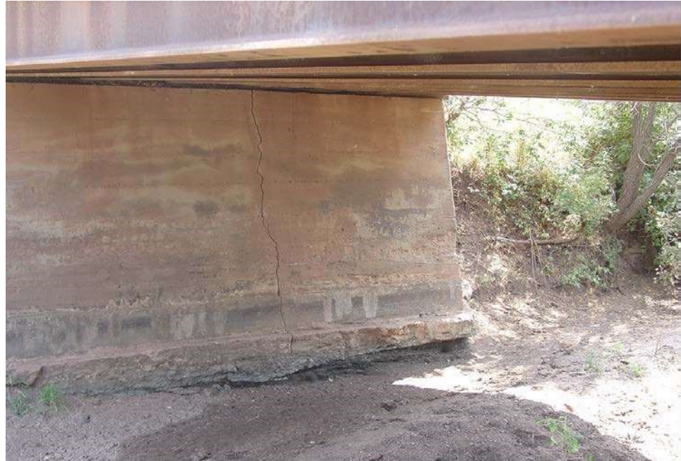
Figure 12.1.41 Crack in Abutment due to Settlement
