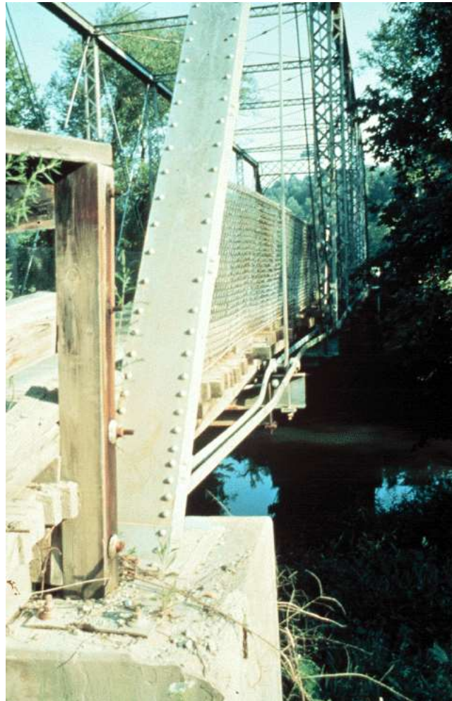
Figure 10.9.22 Buckled Eyebar due to Abutment Movement
