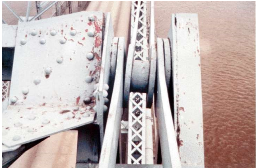
Figure 10.9.24 Asymmetry at an Eyebars Connection
