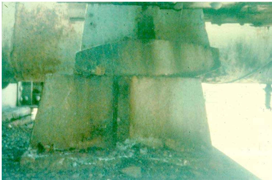
Figure 11.1.29 Rocker Bearing with Excessive Horizontal Movement
