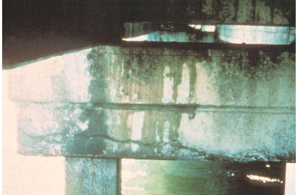
Figure 12.2.31 Crack in Concrete Bent Cap
