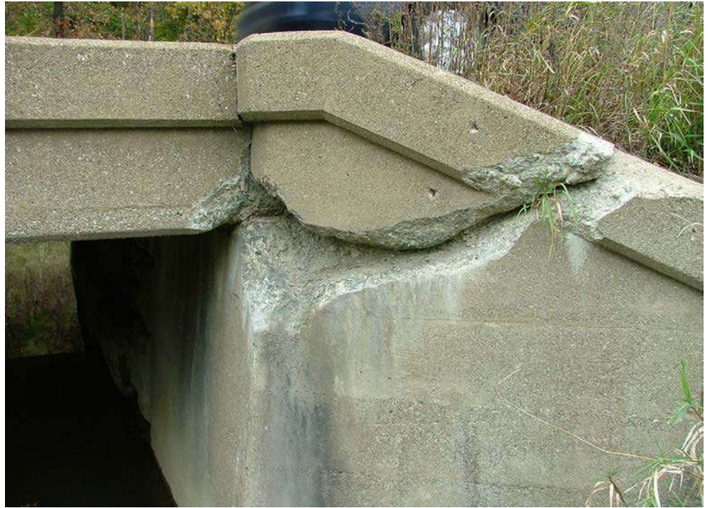
Figure 12.1.32 Spalled Concrete Wingwall
