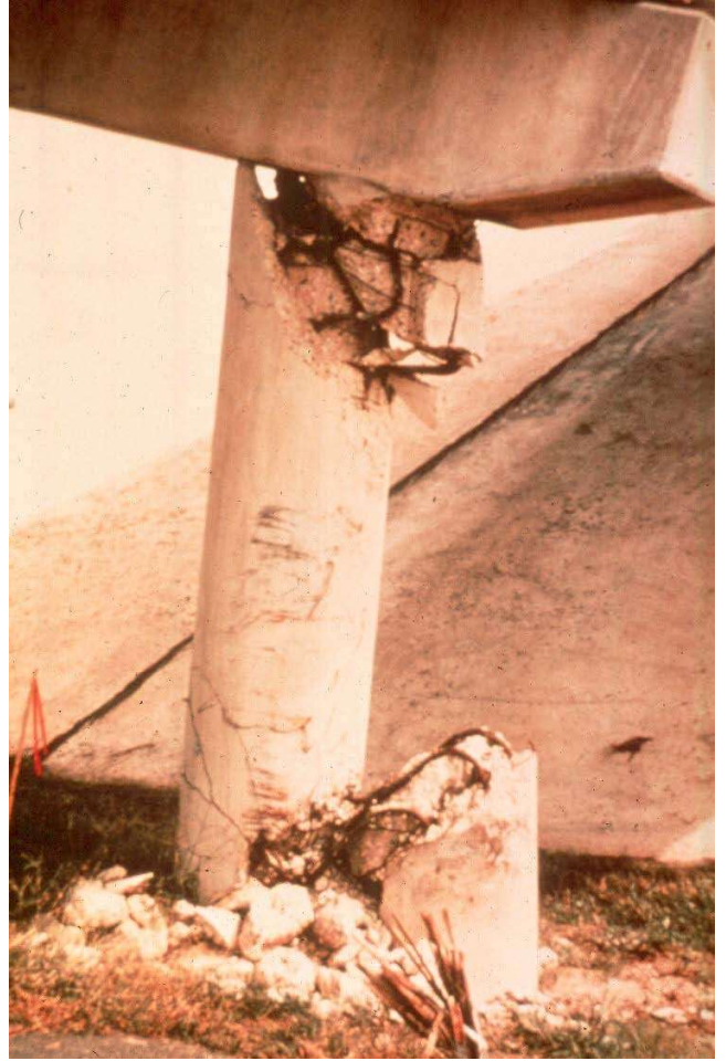
Figure 12.2.33 Collision Damage to Concrete Pier Column
