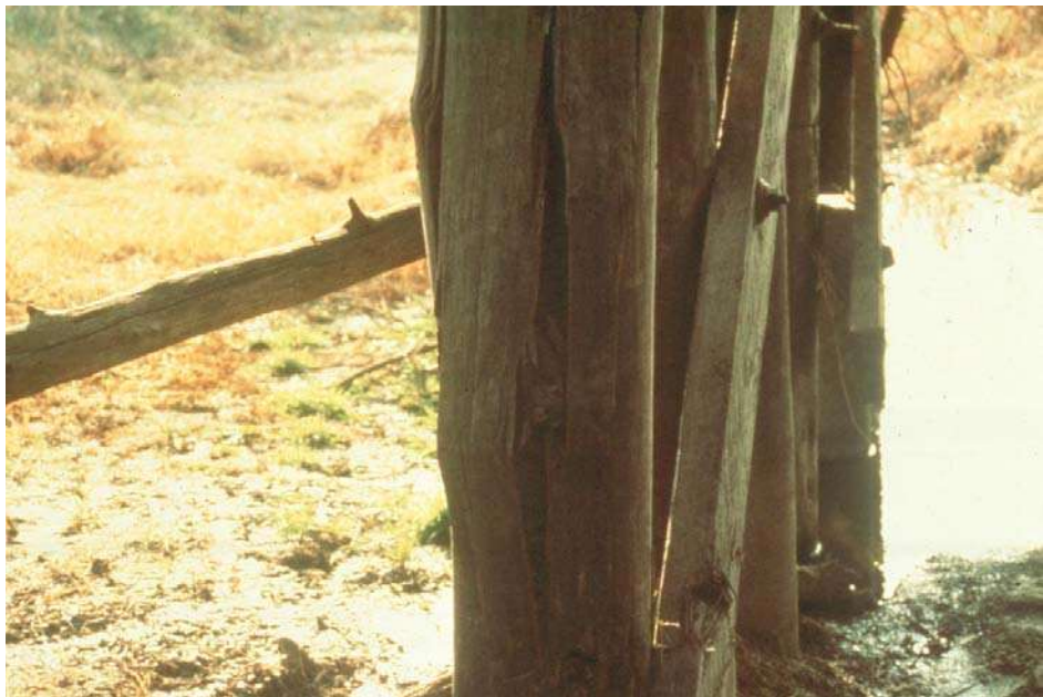
Figure 12.2.41 Timber Pile Bent with Overstress-Partial "Brooming" Failure at First Pile
