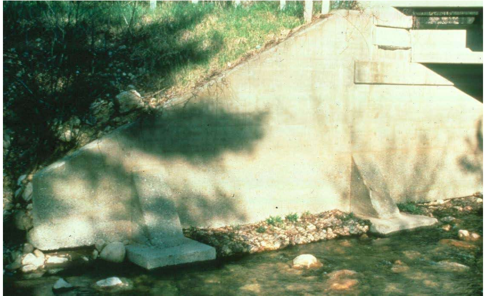
Figure 12.1.52 Scour and Possible Undermining of Concrete Wingwall
