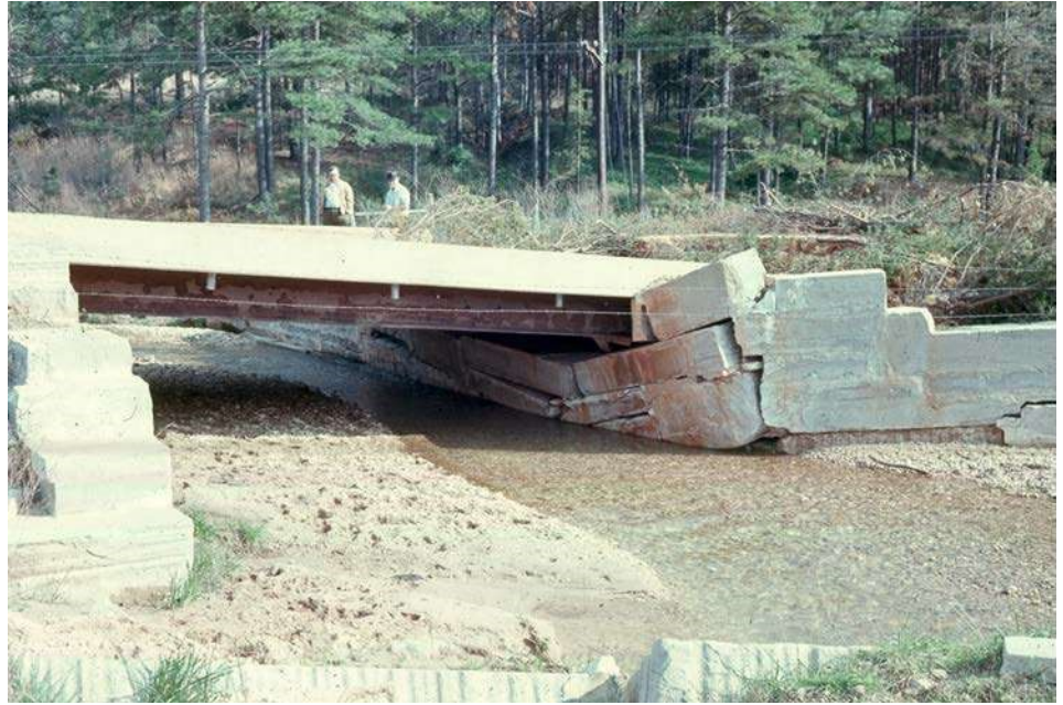
Figure 12.1.50 Abutment with Undermining due to Scour
