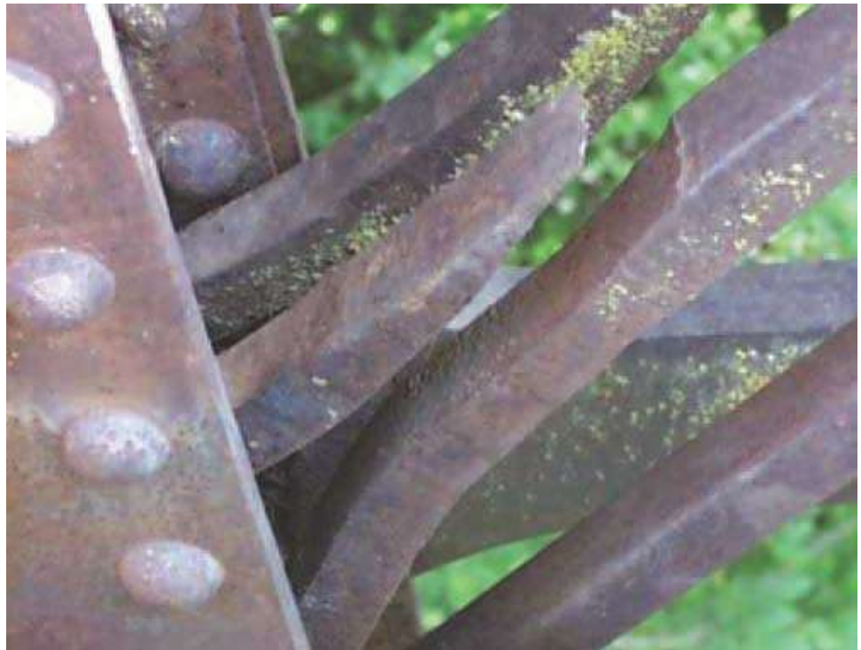
Figure 10.9.20 Forge Loop is Completely Apart
