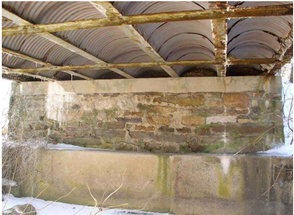
Figure 12.1.31 Cracking in Bearing Seat of Concrete and Stone Abutment
