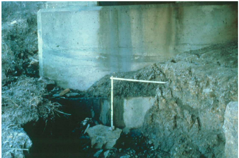
Figure 12.1.45 Erosion at Abutment Exposing Footing
