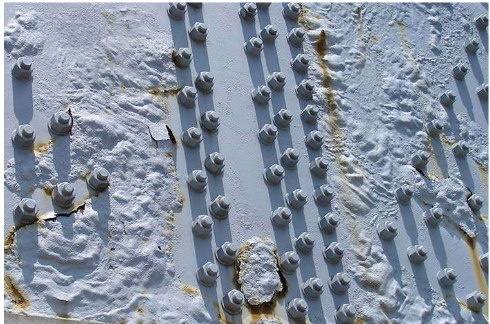
Figure 10.8.28 Gusset Plate with Paint Failure
