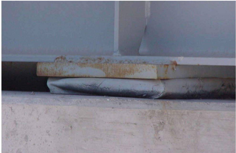
Figure 11.1.40 Neoprene Bearing Pad Excessive Bulging
