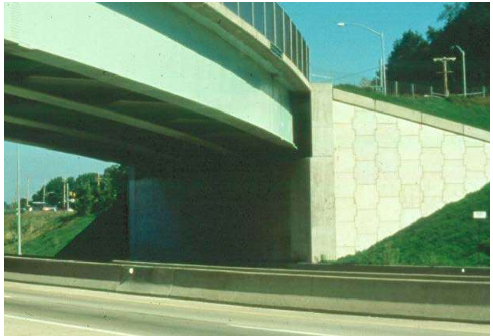
Figure 12.1.28 Independent MSE Wingwall
