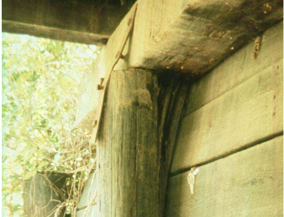
Figure 12.1.37 Local Failure in Timber Pile due to Lateral Movement of Abutment
