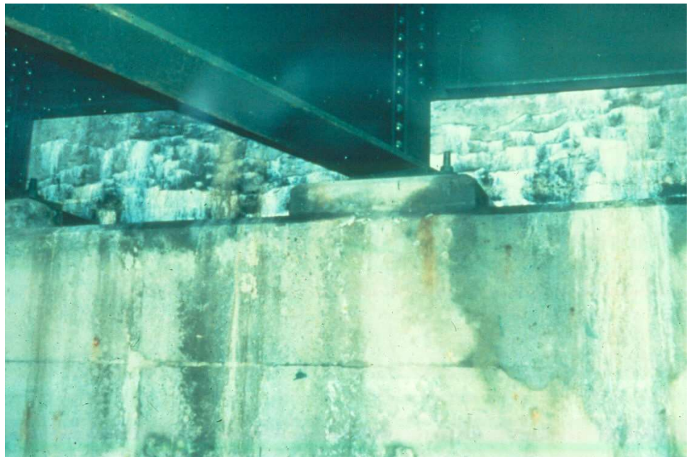
Figure 12.1.33 Cracking and Efflorescence in Abutment Backwall
