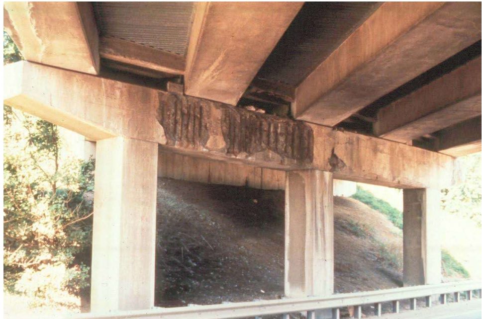
Figure 12.2.32 Concrete Spalling on Bent Cap
