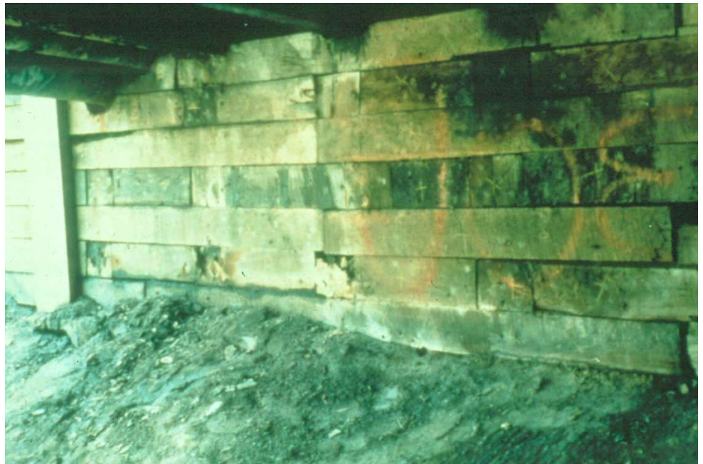
Figure 12.1.36 Decay caused by insects in Timber Abutment
