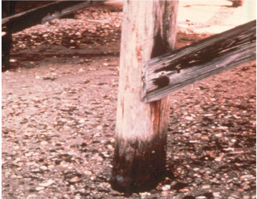
Figure 12.2.40 Decay of Timber Bent Column at Ground Line/Loose Connection
