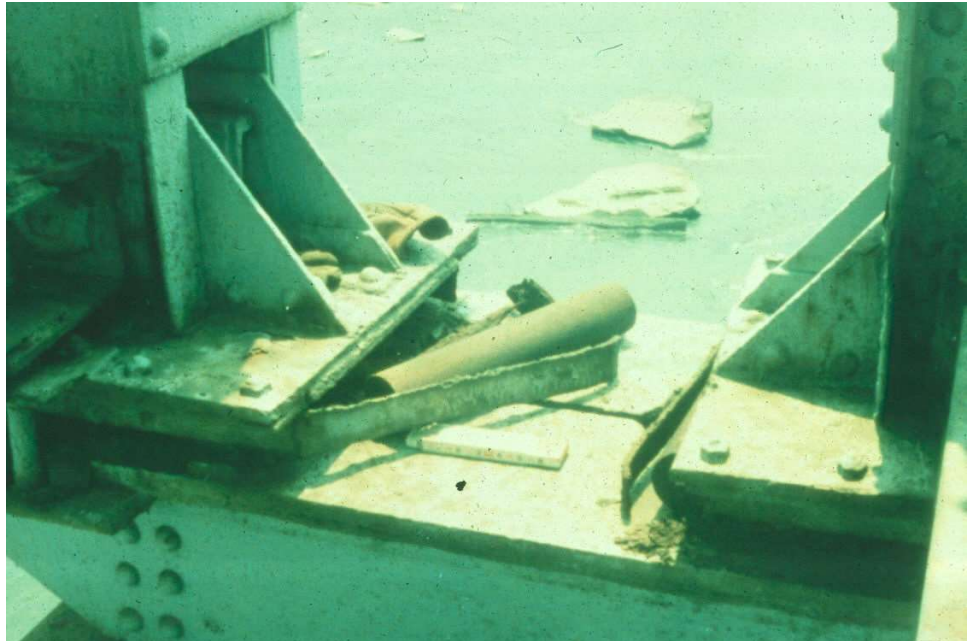
Figure 11.1.34 Damaged Roller Nest Bearing
