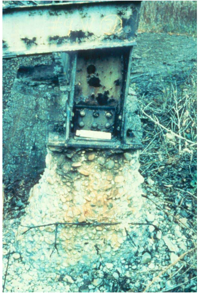
Figure 12.2.35 Deterioration of Steel Bent Leg
