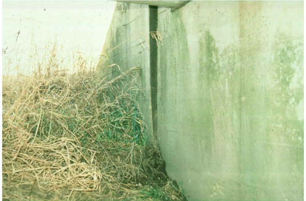
Figure 12.1.49 Rotational Movement at Concrete Wingwall
