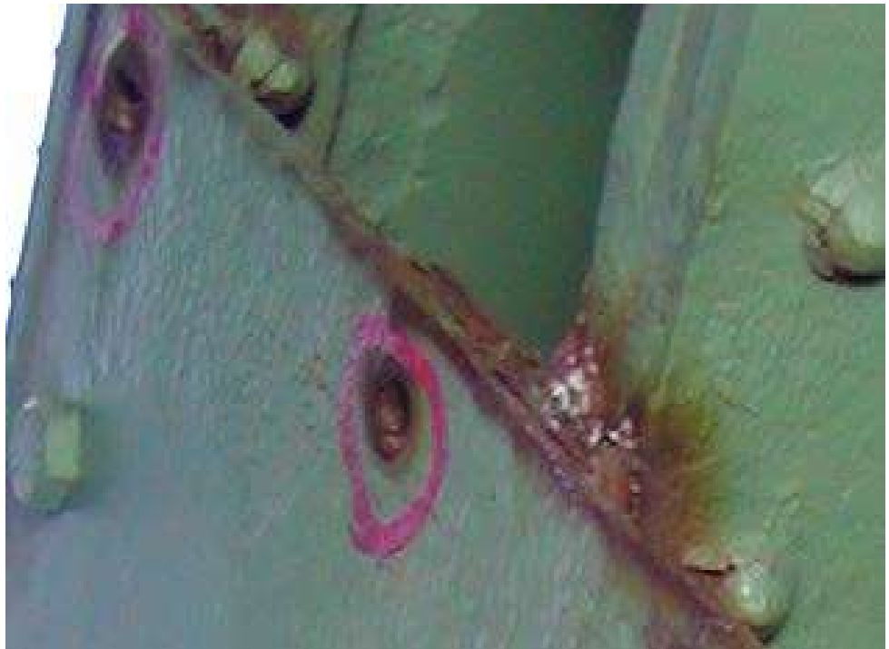
Figure 10.8.29 Missing Bolts on Gusset Plate
