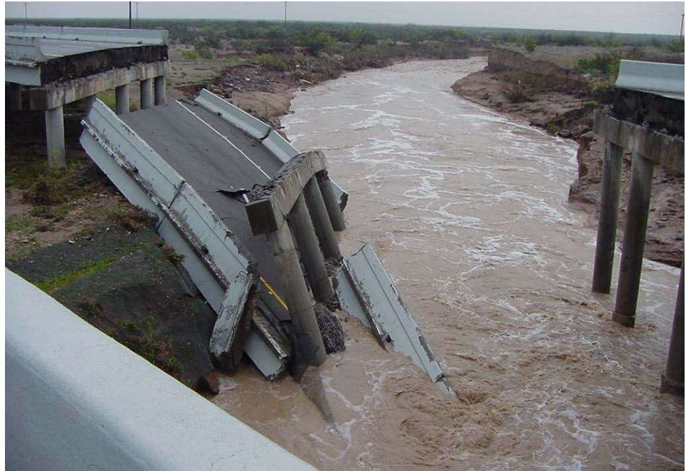
Figure 13.1.3 Pier Foundation Failure
