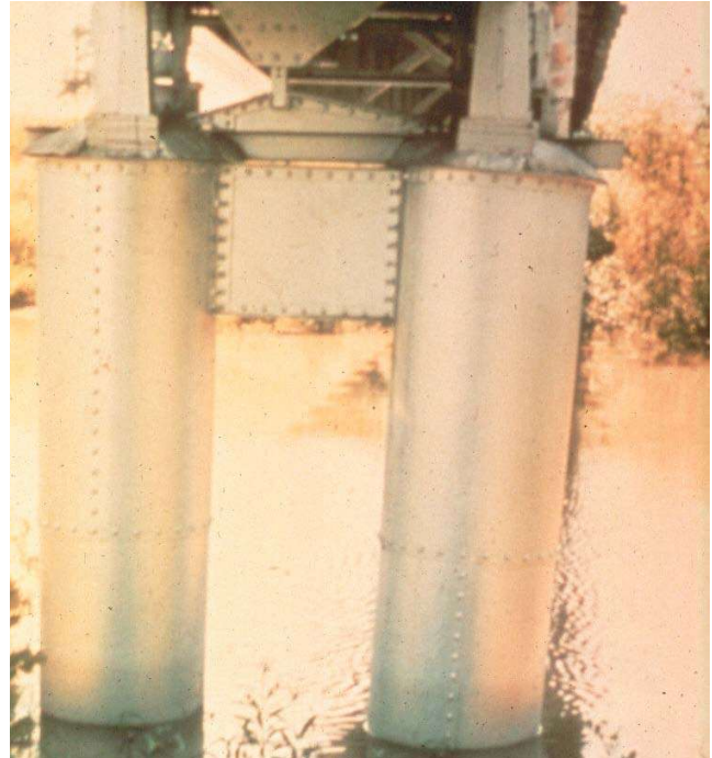
Figure 12.2.49 Tipping of Bent due to Scour/Undermining
