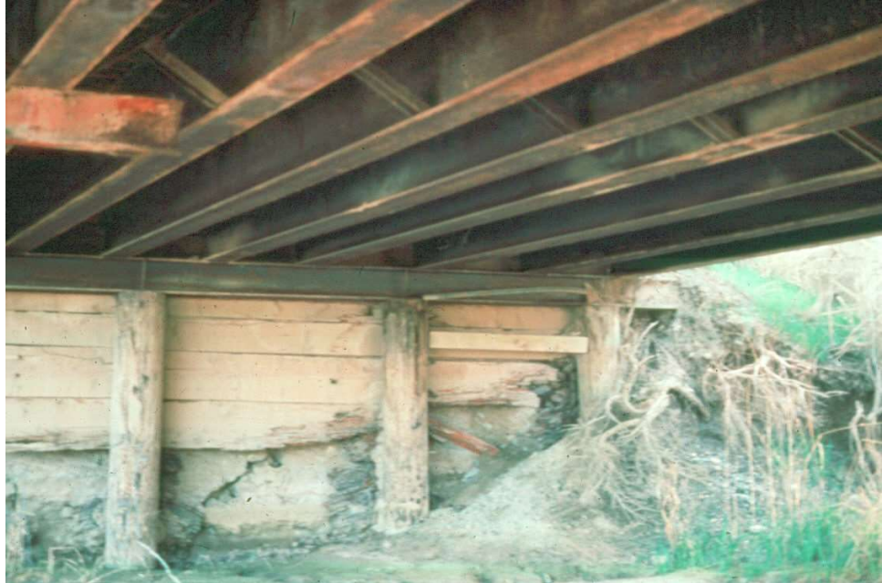
Figure 12.1.38 Decayed Lagging and Abrasion Caused by Scour at a Timber Pile Bent Abutment
