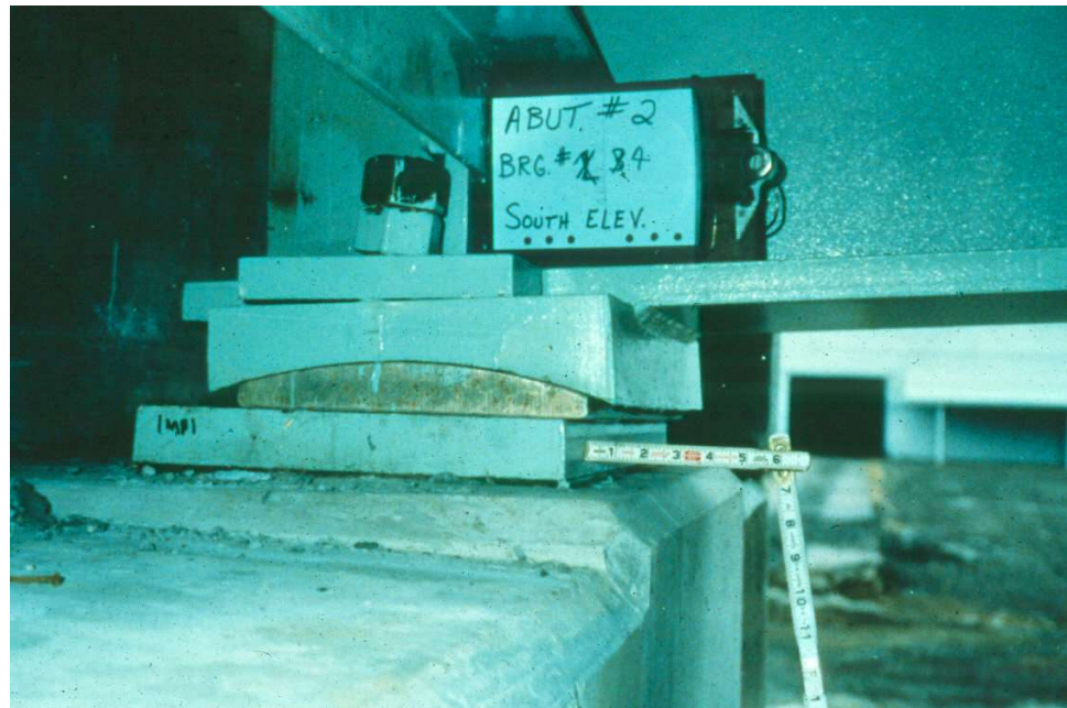
Figure 11.1.32 Longitudinal Misalignment in Bronze Sliding Plate Bearing
