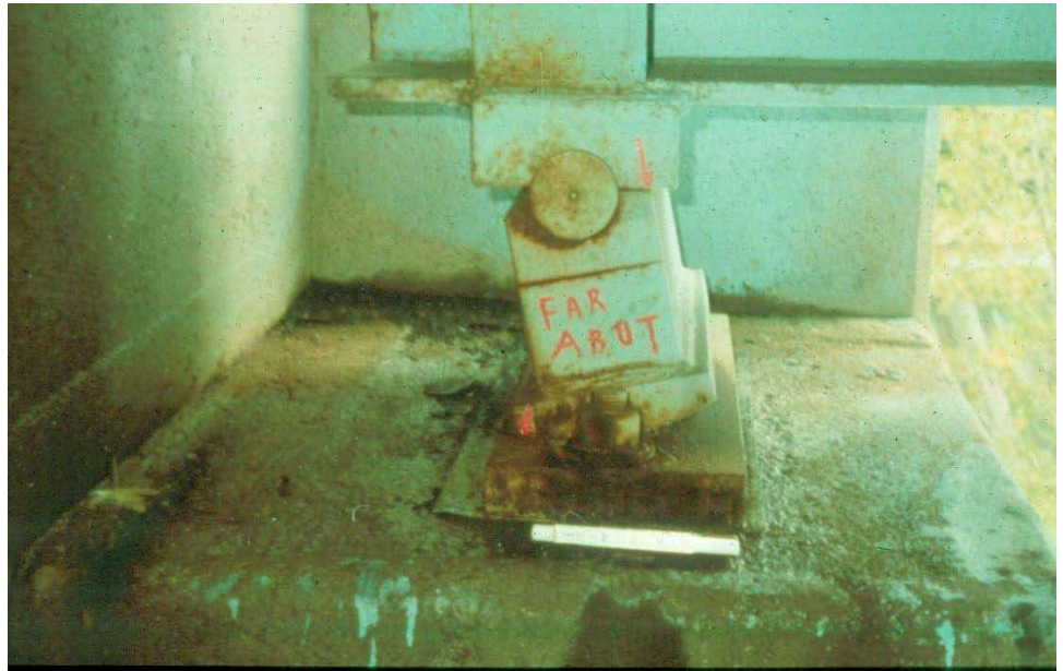
Figure 11.1.43 Broken Pintle on a Bearing
