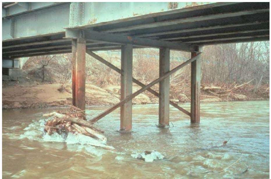
Figure 12.2.36 Corrosion of Steel Pile Bent at Water Surface
