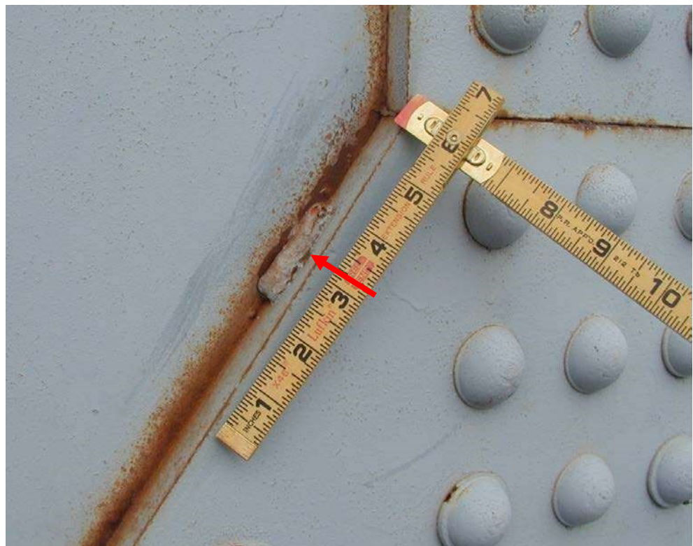
Figure 10.8.26 Partial Length Cracked Tack Weld
