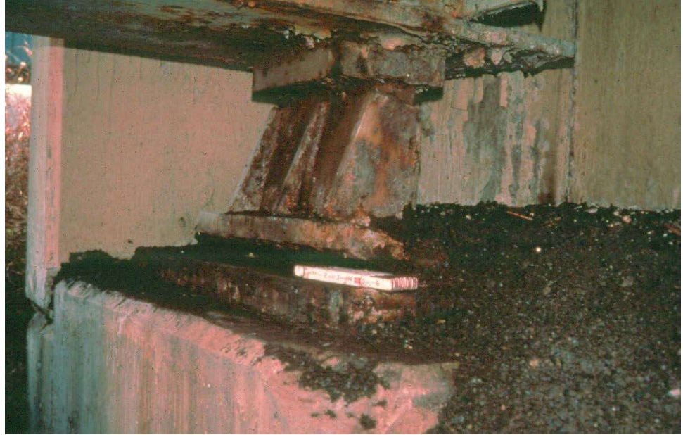
Figure 11.1.28 Heavy Corrosion on a Steel Rocker Bearing
