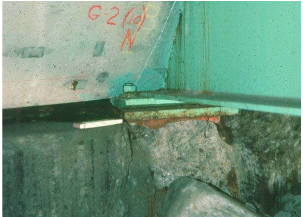
Figure 11.1.26 Spalling of Concrete Bridge Seat Due to High Edge Stress
