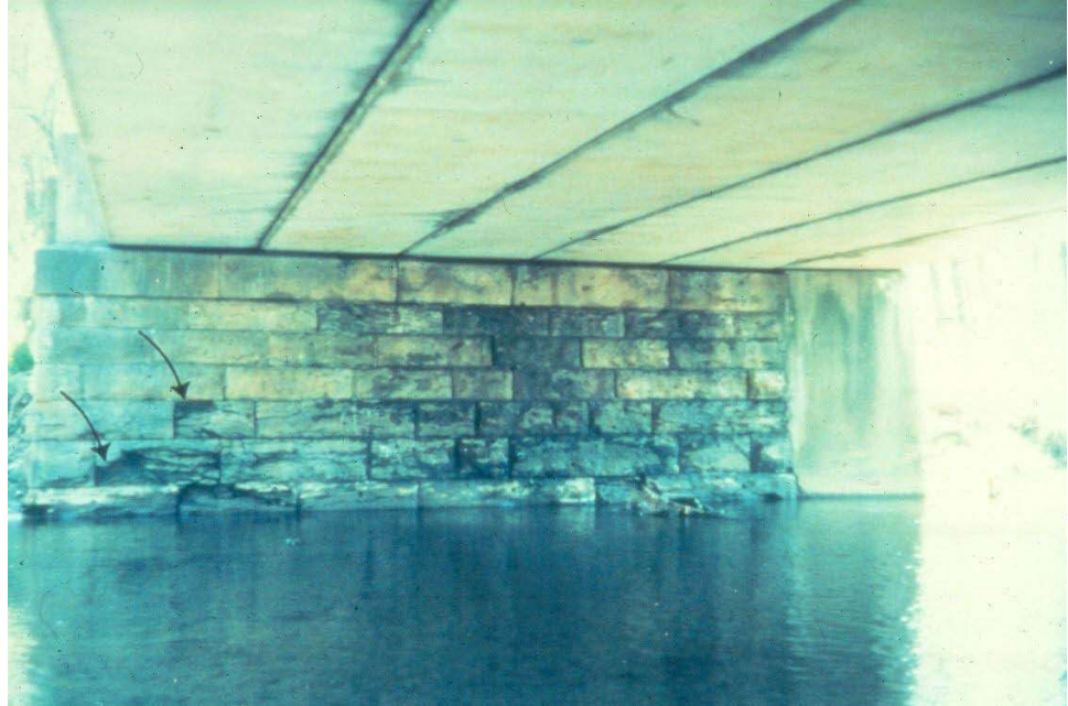
Figure 12.2.34 Deteriorated and Missing Stone at Masonry Pier
