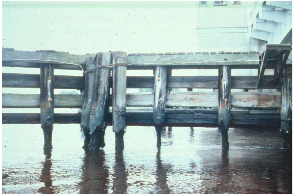
Figure 12.2.54 Timber Fender System with Deteriorated Piles
