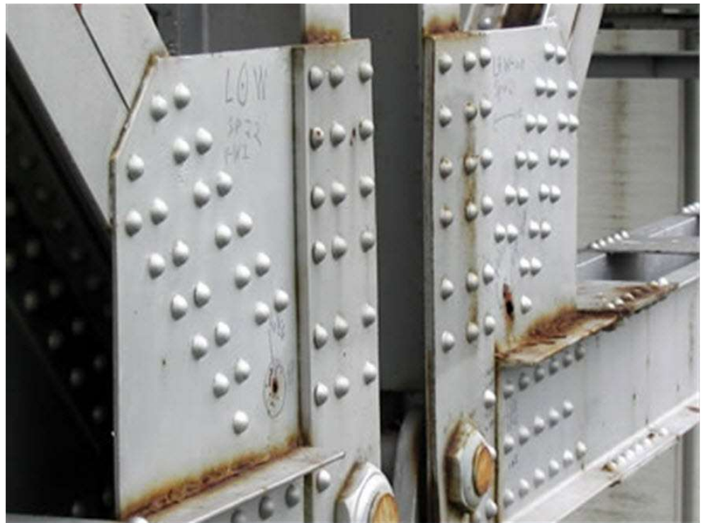
Figure 10.8.17 General Corrosion of Gusset Plates
