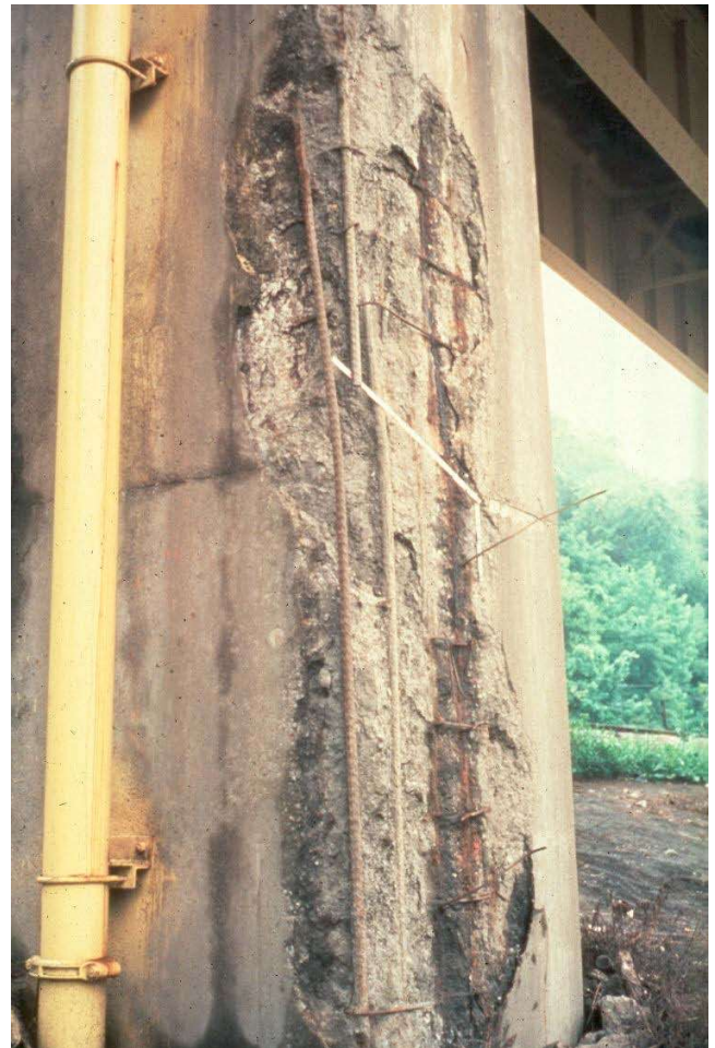
Figure 12.2.30 Concrete Spalling due to Contaminated Drainage
